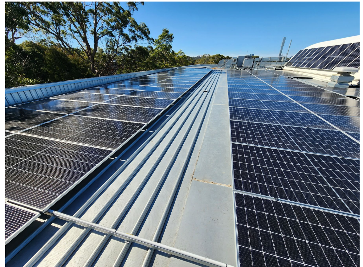
Solar panels at our Lane Cove site in Australia
